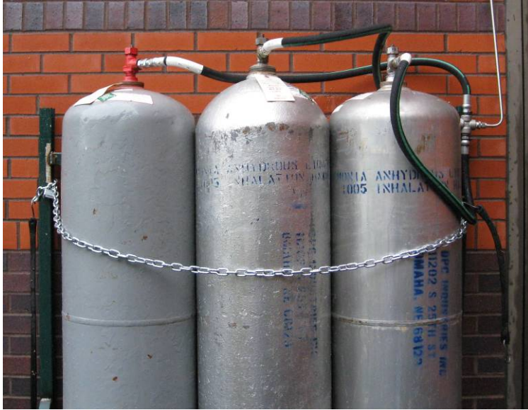
Figure 2 – Ammonia storage tanks.
